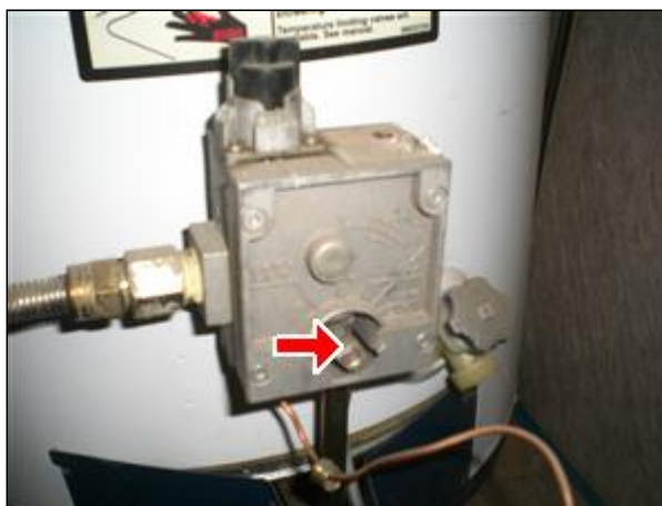
6.2 Picture 2 missing adjustment dial
