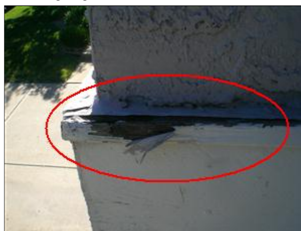
2.0 Picture 5 Trim above garage
