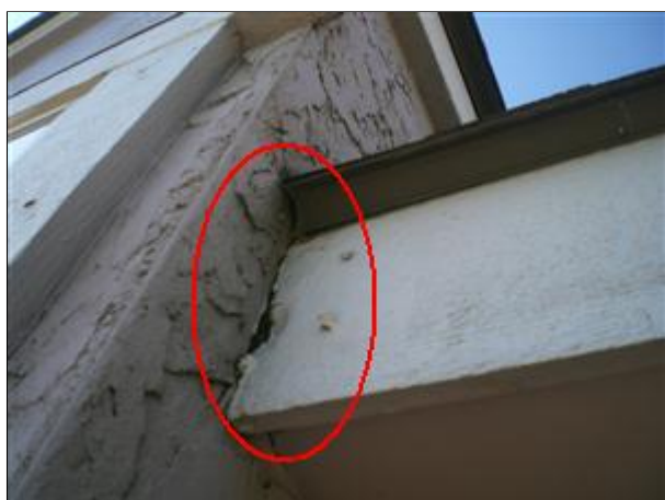
2.0 Picture 3 trim above garage
